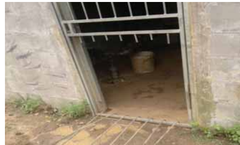
Figure 1.10.2: Oqqabhiyeni generator stolen by cutting a burglar-proof door in Ntambanana
