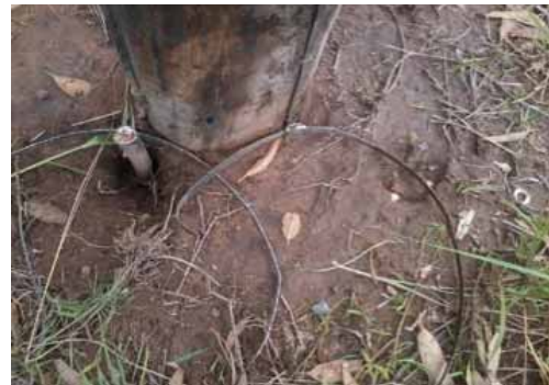
Figure 1.10.4: Electric cable theft at Mvutshini in uMlalazi
